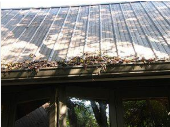
Keep your gutters free of debris so rainwater drains properly. (Photo – M. Waldvogel, NCSU)
