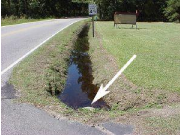
Stormwater run-off and debris in drainage ditches become mosquito breeding grounds. (Photo – M. Waldvogel, NCSU)
